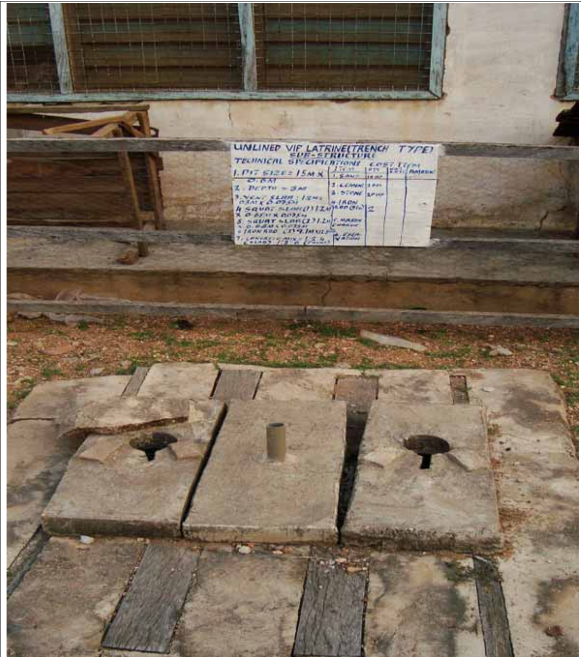
Plate 6: Unlined VIP Latrine (Trench Type)
