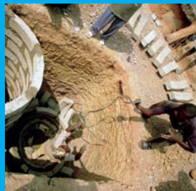
The blocks are built up to form the latrine lining of two latrine pits, within a rectangular pit dug by the householders.
