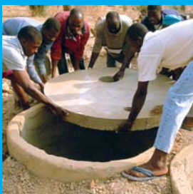
The remainder of the rectangular pits around the latrine pits are filled back in and the latrine slabs are fitted on top of the pits.
