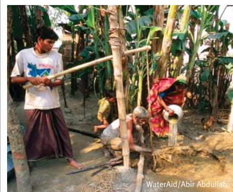
A tubewell being constructed using the sludging method in Erendabari Char, Bangladesh.
