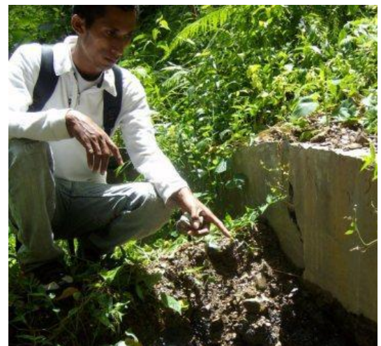
Daniel inspects a cracked intake
