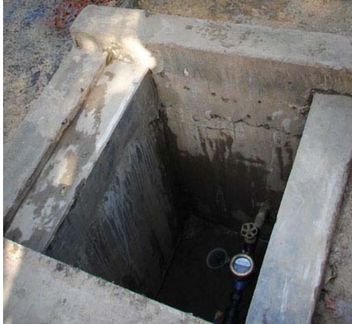
The water meter
