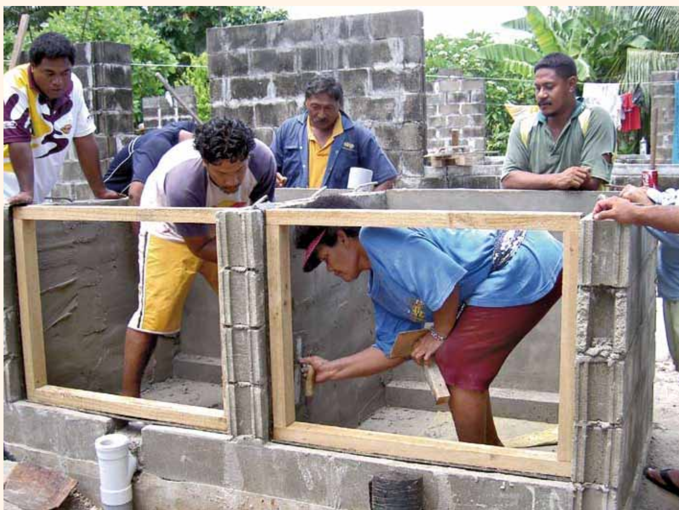
Trainees around the composting toilet in Tuvalu. The trainee woman doing rendering represents Funafuti Women's Group and plans to seek funding to run a similar training for women (who have never done any building before). Watching her is the carpenter from Public Works, the Senior Health Inspector, and a guest trainee from Ministry of Health in Kiribati, which has led to immediate mobilisation of resources for replication of the training in their country. Photo: Leonie Crennan
