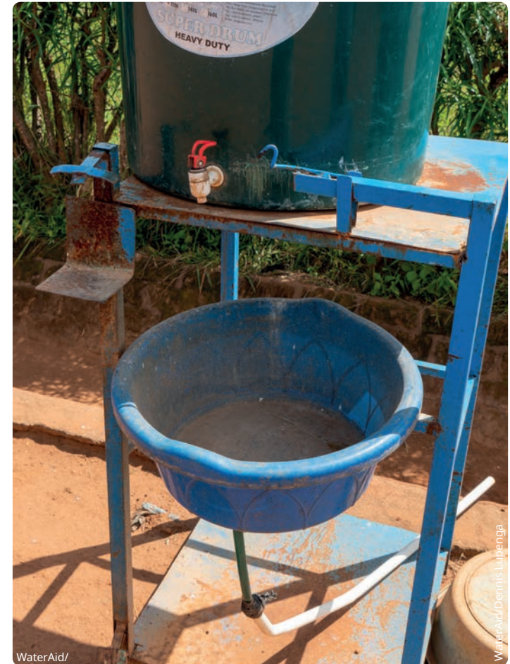
▲ A handwashing station with no water, Mkunzi Health Centre, Ntchisi district.
