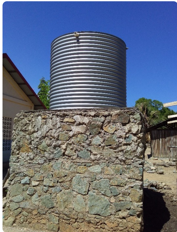
Figure 7 – The water tank at the Ediri primary school is typical of many of the school water tanks in Liquiçá. (Liquiçá Municipal Department of Water Supply, Sanitation and Environment/Herminio Soares)
