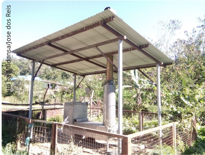
Figure 12- Incinerator at the Turisca community health centre
