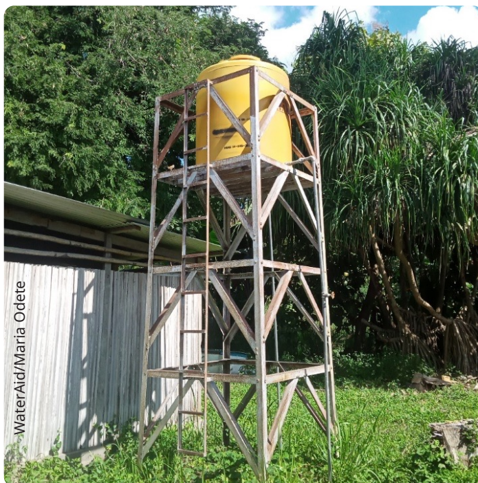
Figure 5 - While the Uma Berloic Health Post water supply meets minimum basic JMP, the generator and pump require rehabilitation to maintain this service into the future.
