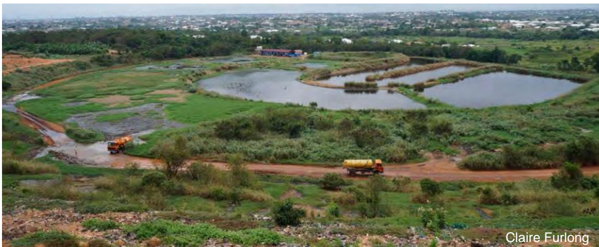
Picture 2: Dompouse faecal sludge (septage) treatment plant
