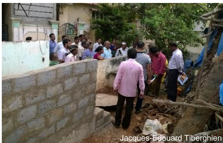
Early-bird visit of GVMC Commissioner and GVMC staff monitoring the construction of a household toilet.
