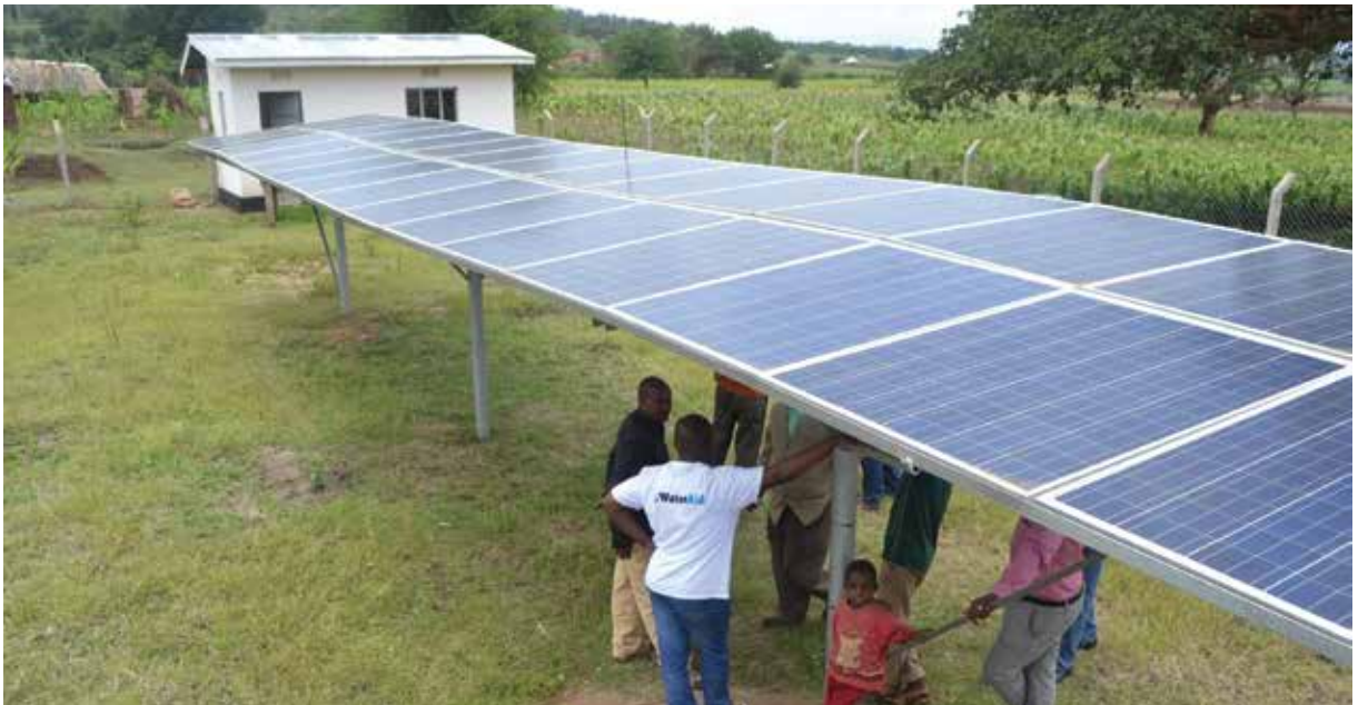
A solar powered water and sanitation facility constructed by waterAid in Tanzania.
