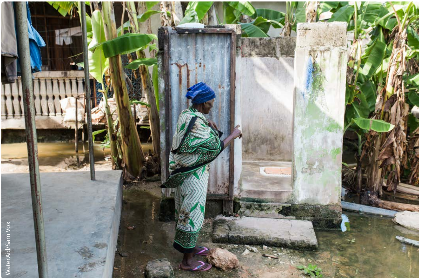
● Teodora shows how recent floods have infiltrated the water storage tanks and the pit latrines. This has reduced her access to a toilet and means she will have to come up - at least temporarily - with a new way to access safe drinking water. Kigamboni, Tanzania. January 2020.
