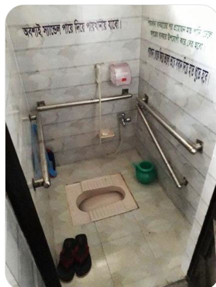
Improved WASH facilities
