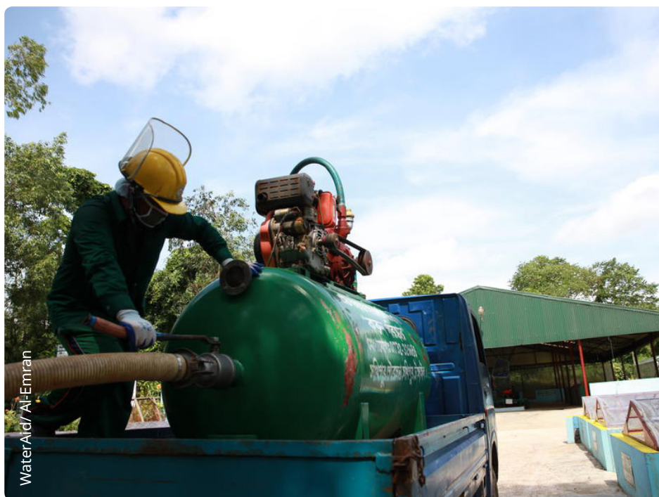
▲ Fig.5: A worker prepares to empty a Vacutag sludge pump in Sakhipur
