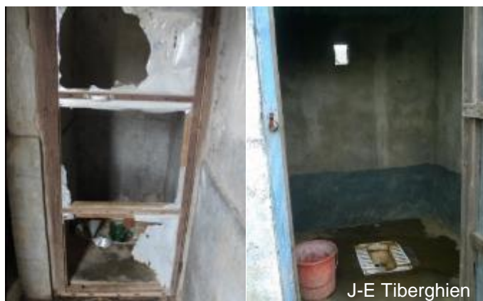
Figure 1: Latrine blocks at Kaiika lower secondary school, Padam Pokhari, Makwanpur district. Credit: Jacques Edouard-Tiberghien.
